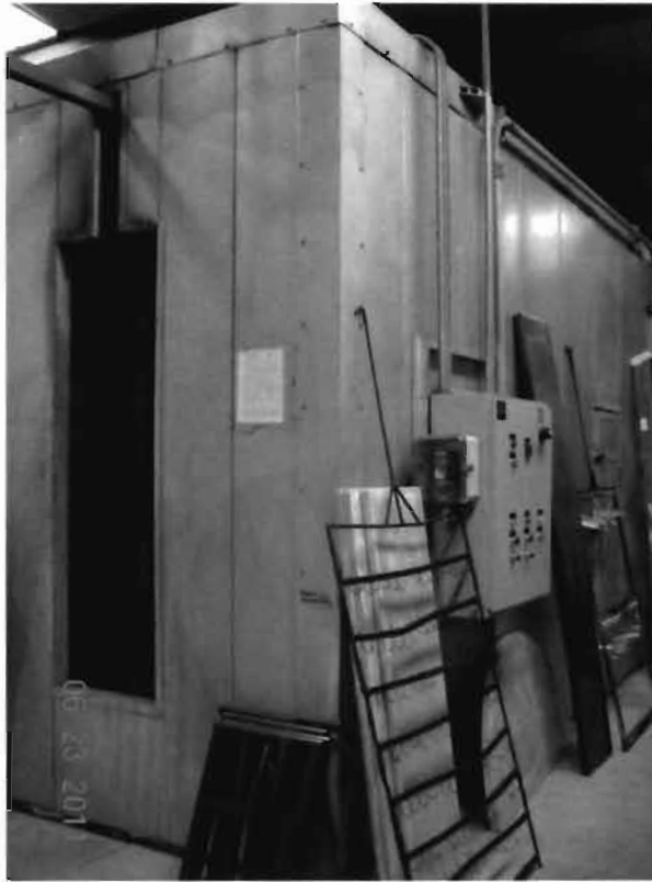
Photograph of Dry-Off Oven (Located Inside Plant)
