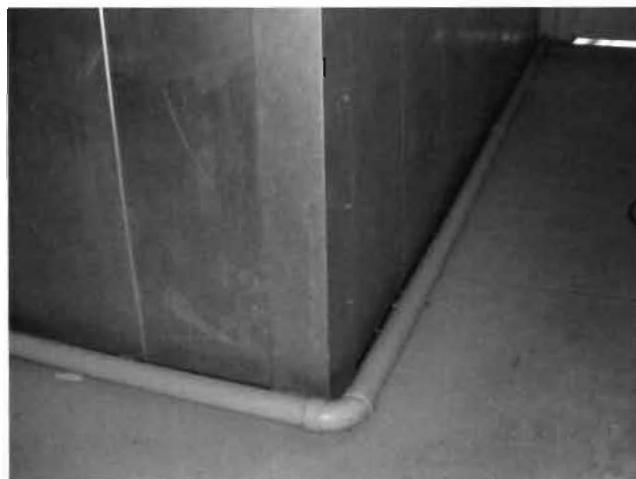
Photograph of PVC Process Water Line Located on Plant Floor Clearly Visible For Inspection
