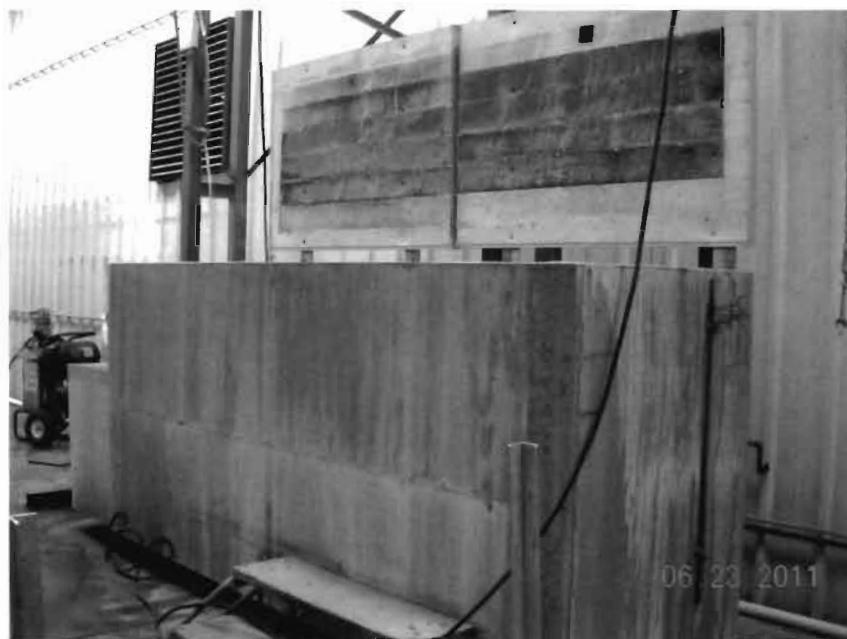
Photograph of Dip Process Tank Located Under Cover (Capacity: 1000 Gallons)
