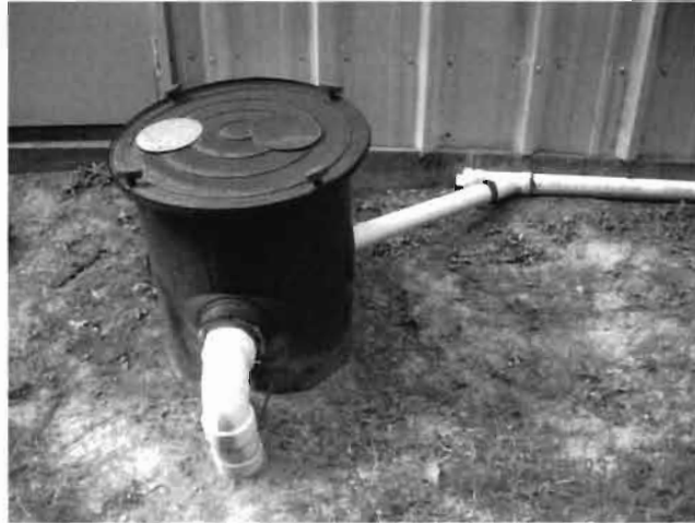
Photograph of Process Water Collection Fixture Where All Process Water Lines Commingle Prior to Entry into Municipal POTW - Located on North Side of Building
